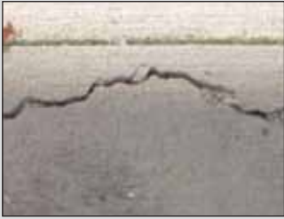
1. The Garden Centre developed shrinkage cracks parallel to the control joints ranging from hairline to 6mm wide.
