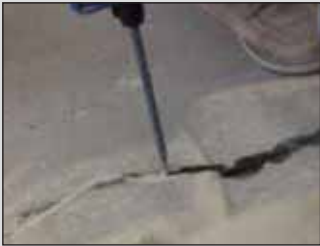
5. Additional material and sand is added to fill the crack up to the top.
