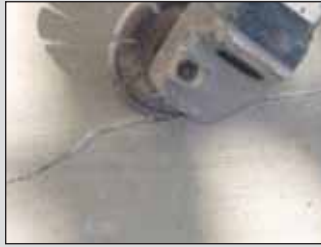
2. The cracks are lightly scored and cleaned out with a diamond blade attached to an electric grinder. Dust and debris is removed with a vacuum.
