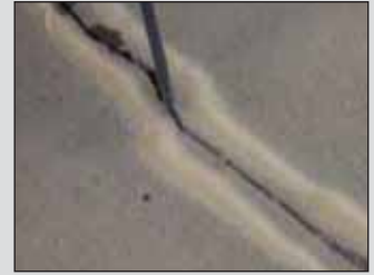
4. Repairs are made full depth. Silica sand is added to stop "sinkers" and build a polymer concrete matrix.
