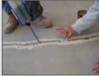
3. Ultra penetrating Roadware 10 Minute Concrete Mender™ is applied directly the crack followed by a 6mm layer of 10 Minute Silica Sand.
