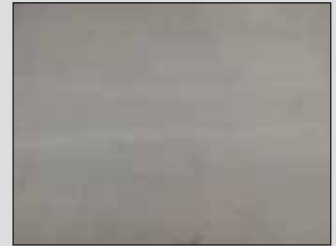
8. After the repair cures for an hour, the crack is repaired structurally, and is nearly invisible.
