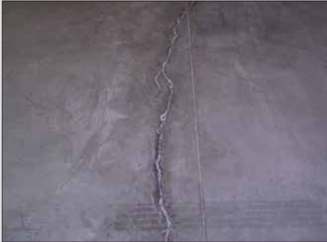
Crack in a newly laid carpark floor
