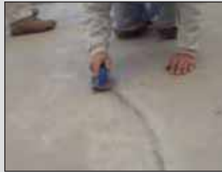
7. After 10 minutes at 22°C, the repair is ready for traffic or finishing if desired. Here a concrete finishing stone is used to blend the repair with the surrounding concrete.
